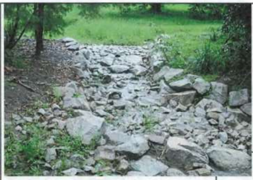
Example of buffered outfall with coarse aggregate (Catchments and Creeks Pty Ltd., 2020)
