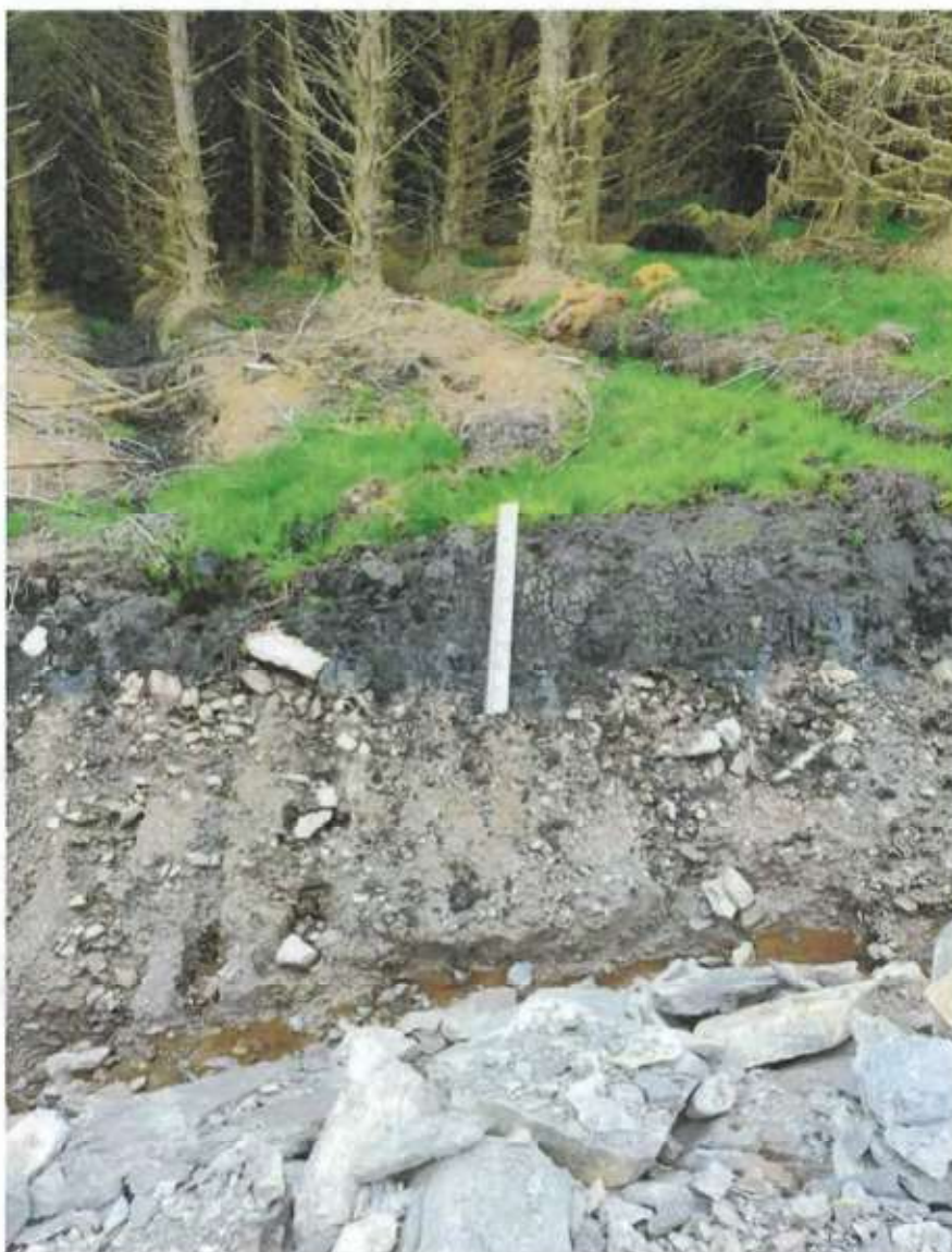
Peat and fill exposed at new access track and drainage associated with ongoing forestry activities observed during site survey.
